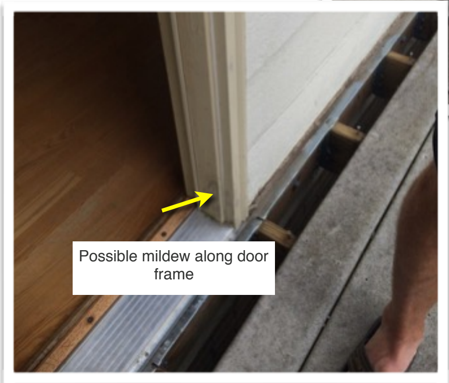
Possible mildew along door frame
